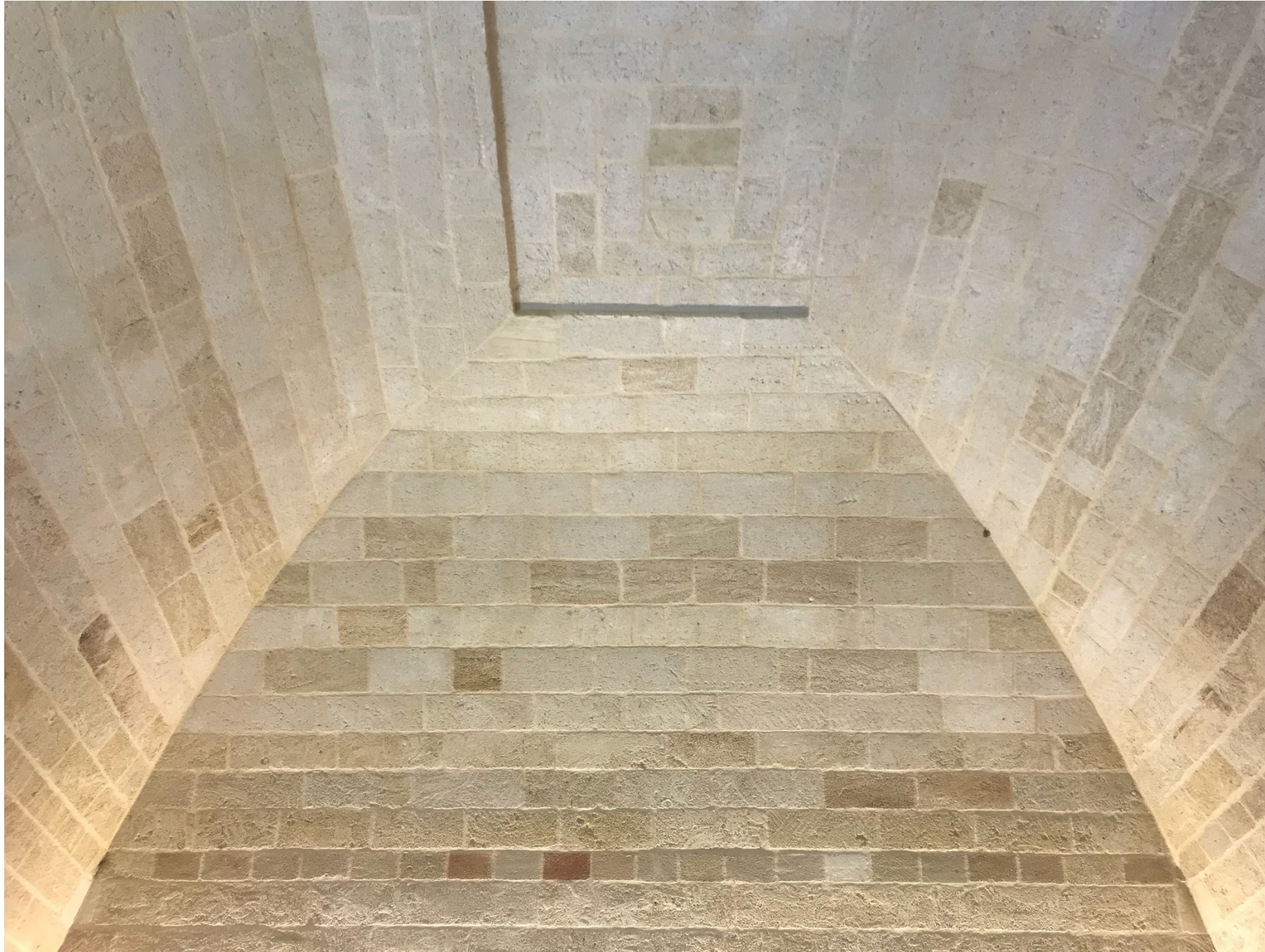
Pavilion vault with square plan, Otranto, Italy
