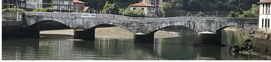
Fig. 1. The effect of soil settlements on the Deba bridge (Spain): a clear subdivision of the structural domain into rigid macroblocks can be seen.
